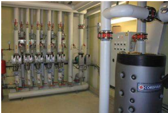
Fig. 3. Technical room (MORBIHAN ENERGIES).
